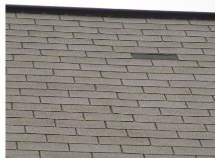
Figure 4: An example image from a roof survey that would get a positive label for the “missing shingle” label in our experiment.
